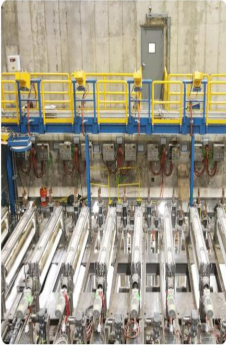
Endless Strip Production induction furnaces
