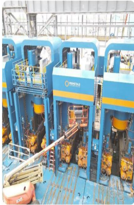
Endless Strip Production roughing mill
