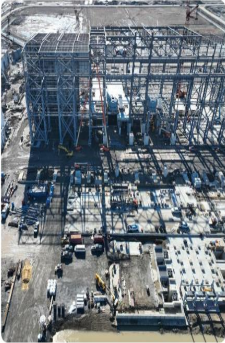
Electric Arc Furnace steelmaking plant
